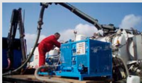
Transferring the sludge via the DOD to the AVC dewatering container.
